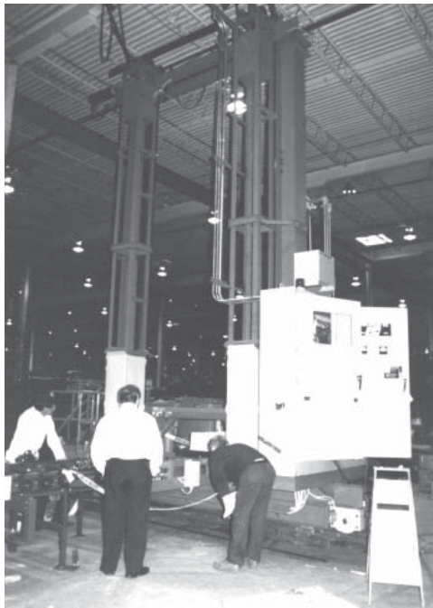
ASRS being set up and tested in the plant. This system feeds drying ovens in a mold process.
